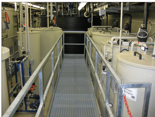
Figure 4: Bioreactors with sedimentation chambers (Katharinen Hospital, Stuttgart, Germany) [EnviroDTS]
