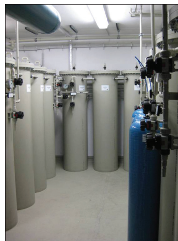
Figure 5: Overview of the adsorption filter modules with modified activated carbon (Katharinen Hospital, Stuttgart, Germany) [EnviroDTS]
